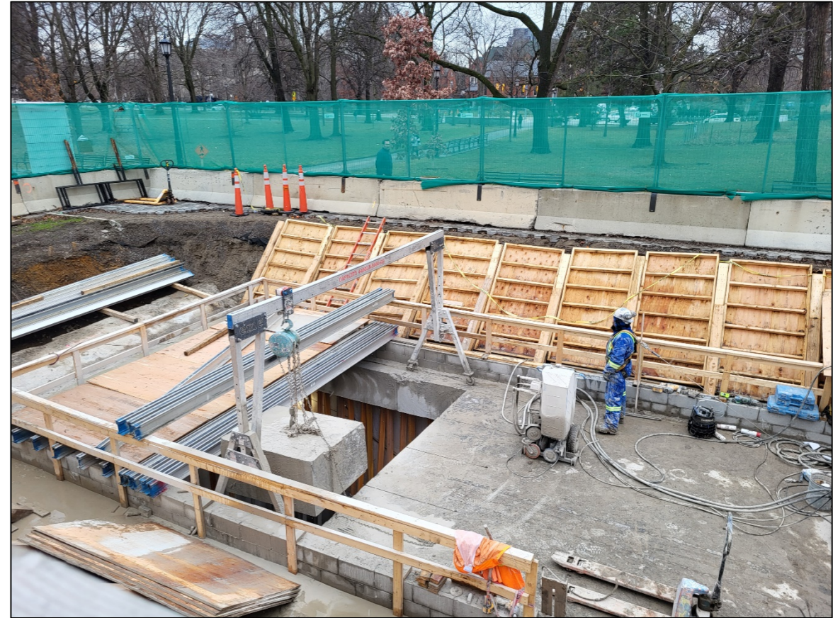
Cutting the tunnel roof at south end of Museum Station for the Second Exit/Entrance in Queen's Park Circle, looking west.
