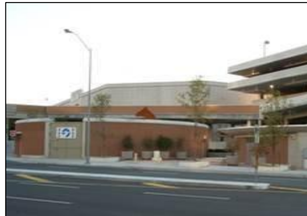
Exhibit E4-3: Traction Power Substation Don Mills Station
