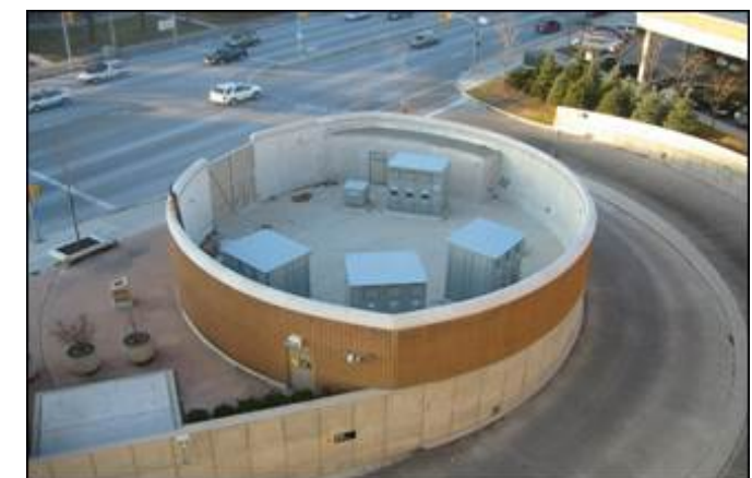
Exhibit E4-4: Traction Power Substation Aerial View
