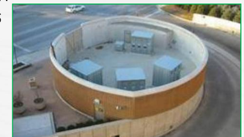
Example Traction Power Substation
