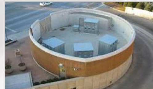
Traction Power Substation
