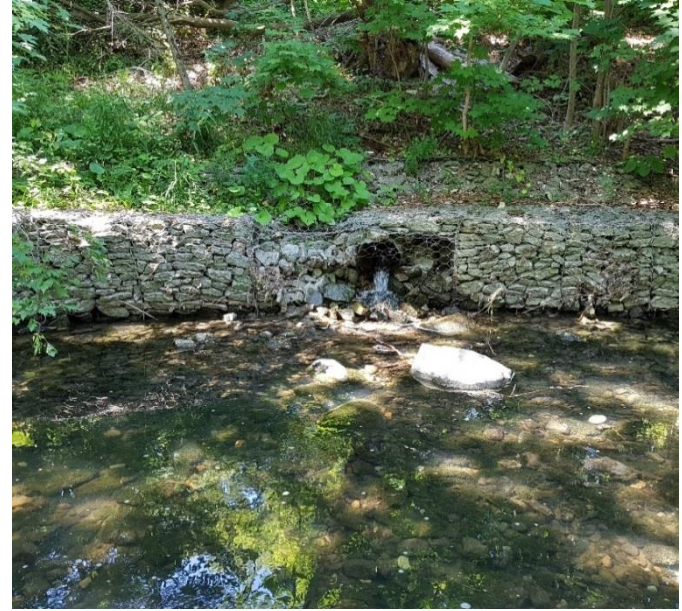
Photograph 14 ↑ Reach 2 Gabion baskets failing along the left bank, looking southwest
