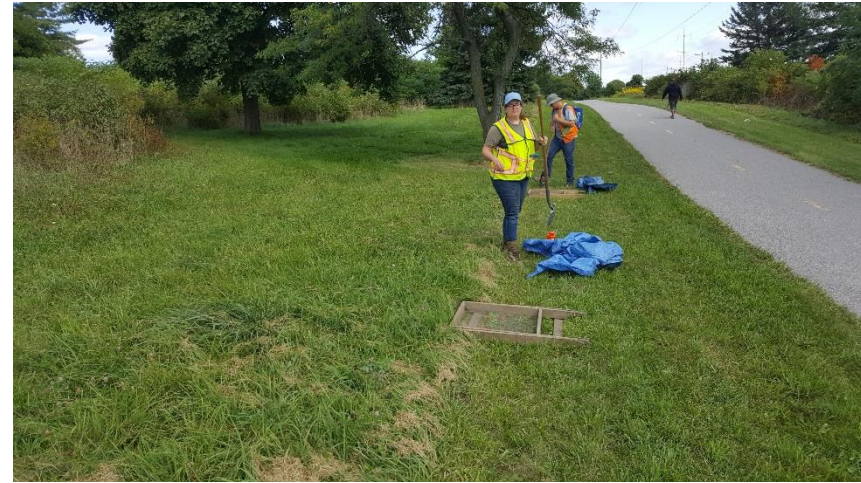
Photo 11: Crew at work test pitting within the Gatineau Hydro Corridor, east of McCowan Road for TPSS 2; view northeast
