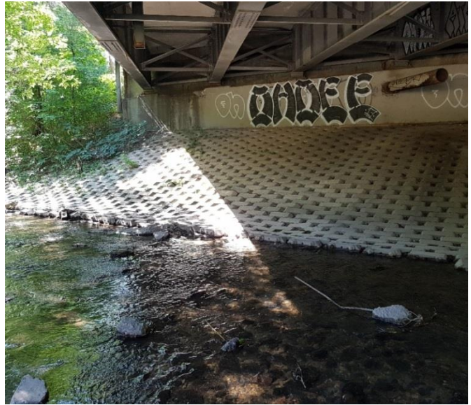
Photograph 2 ↑ Reach 1 West Highland Creek, looking towards the interlocking brick bank at the McCowan Road bridge
