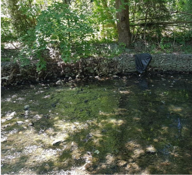
Photograph 13 ↑ Reach 2 Gabion baskets failing along the left bank, looking upstream
