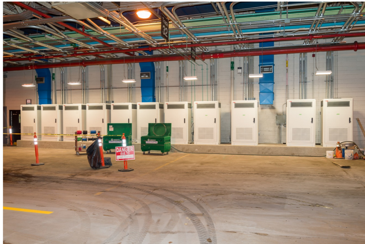
Photo of e-bus charging stations (power and controls) at Mount Dennis Garage
