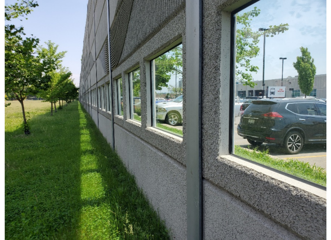
Current Mount Dennis Garage parking lot with noise wall. Noise wall to remain.
