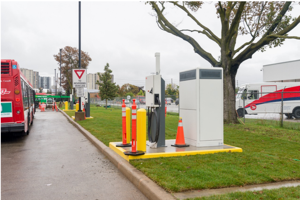
Photo of e-bus charging station at Mount Dennis Garage
