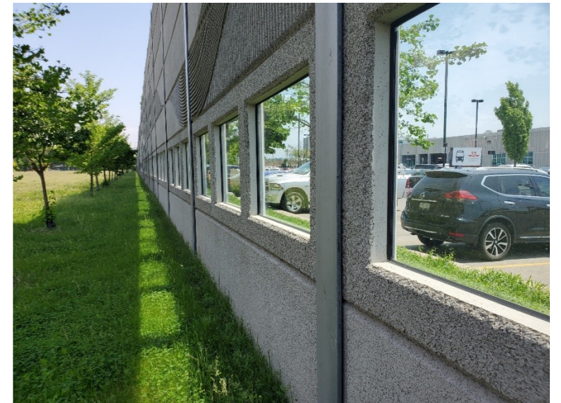
Current Mount Dennis Garage parking lot with noise wall. Noise wall to remain.
