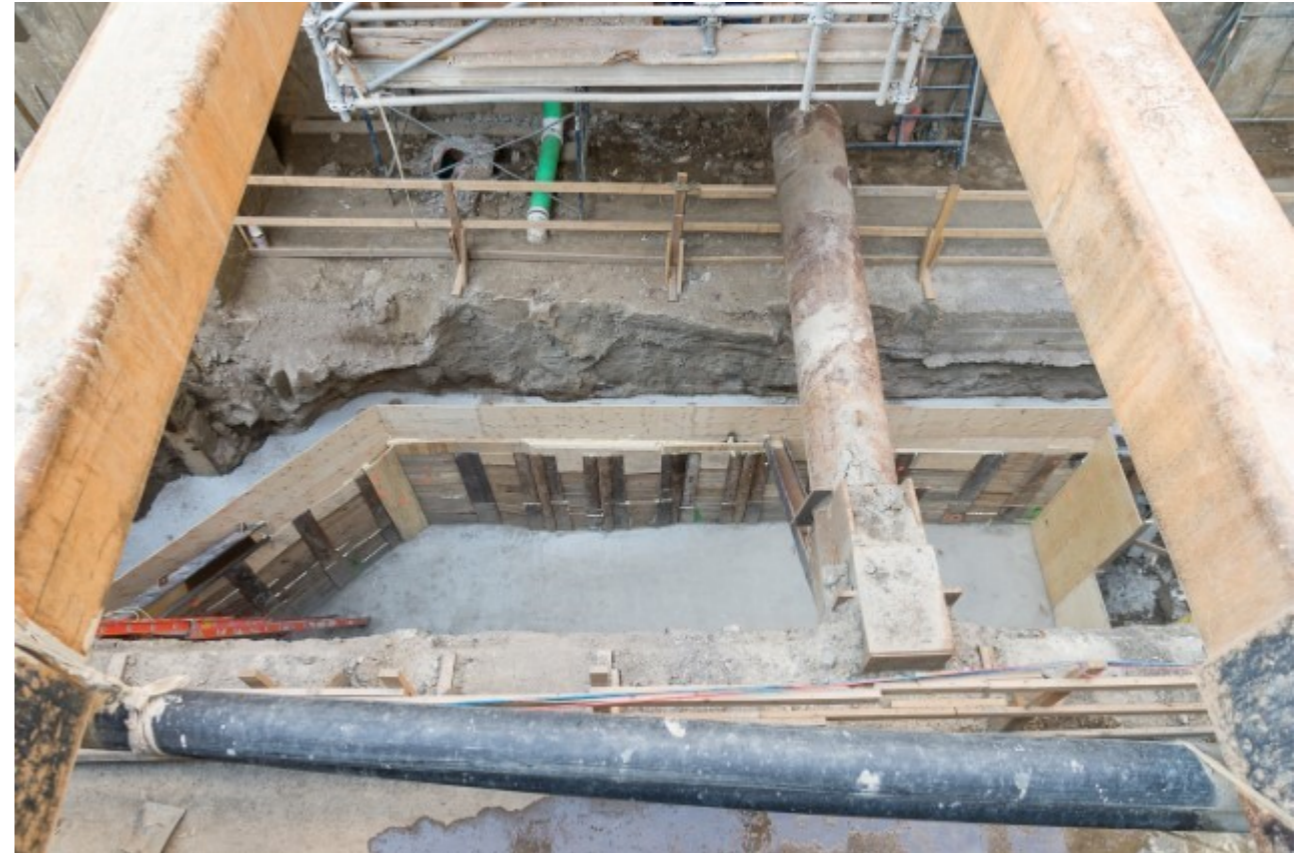
Photo of: Mud slab at the south end excavation to aid in the development of new concourse and stairs from platform level.
