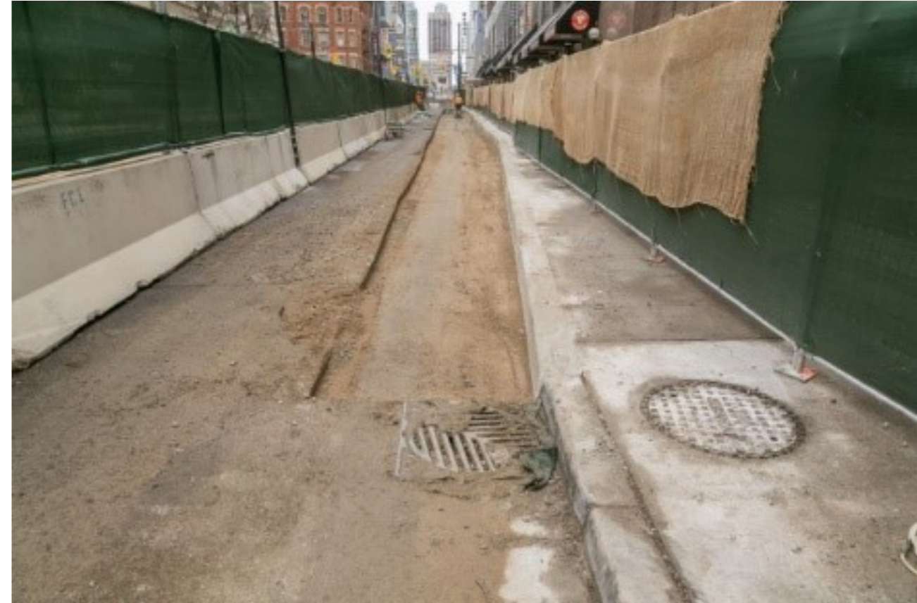
Photo of: Site enclosure where a portion of Yonge St. is closed in order to stage construction.
