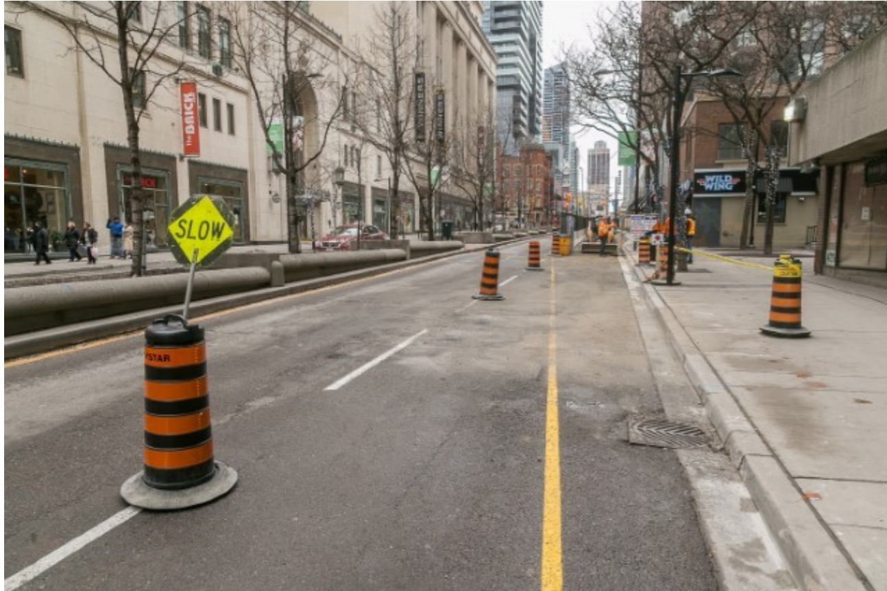
Photo of: Staging traffic for workers to access the site to complete curb work.
