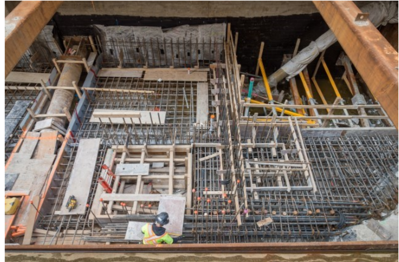
Photo of: Formwork and rebar around elevator pit – to be poured with concrete.
