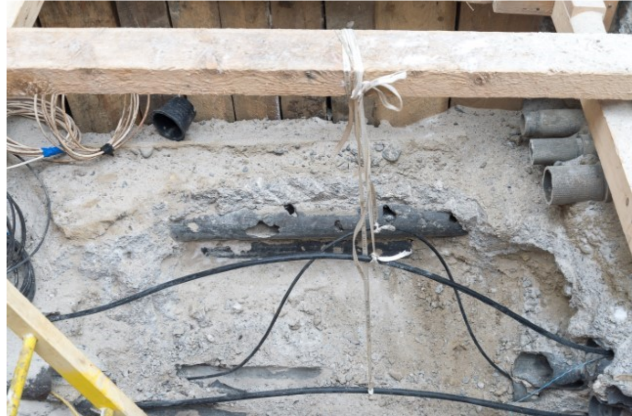
Photo of: Exposed duct banks to be rerouted below ground – exposed conduits to be reattached and fitted with utilities such as telecommunications, internet, electrical etc.
