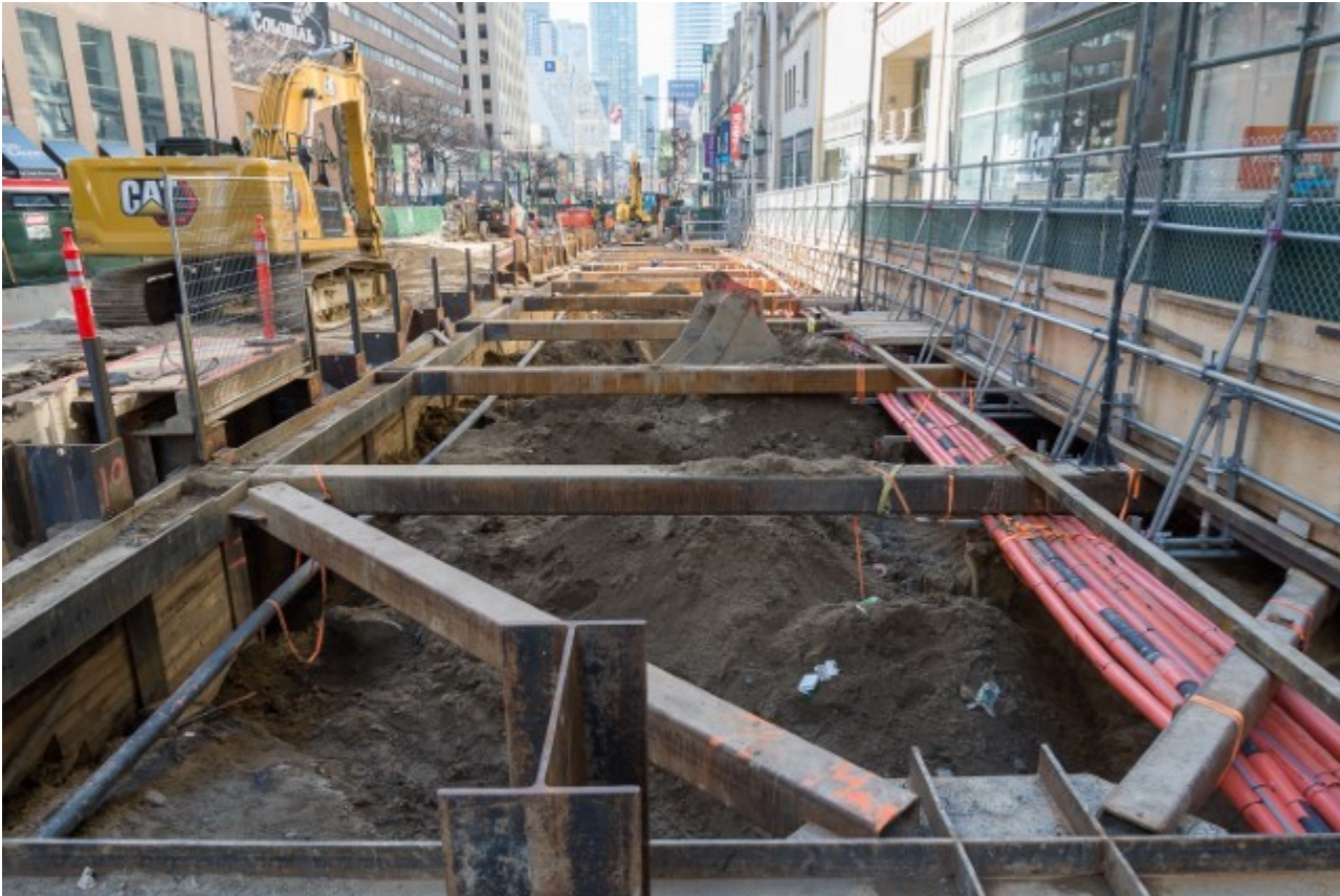
Photo of: Walers, struts and horizontal hollow steel section beams in order to support shoring for further excavation.
