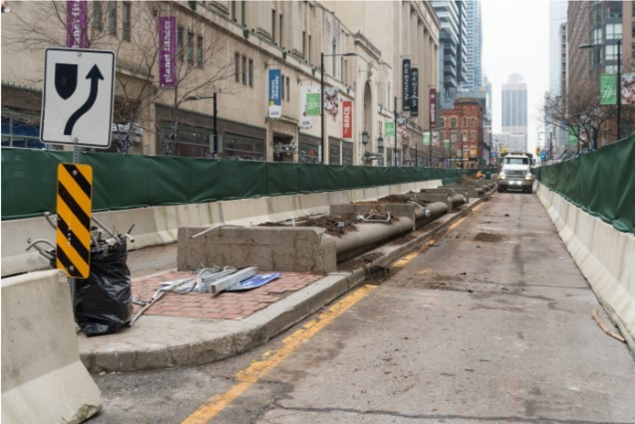
Photo of: Median Demolition – median to be removed down Yonge St. in order to start Stage 2 demolition and excavation.
