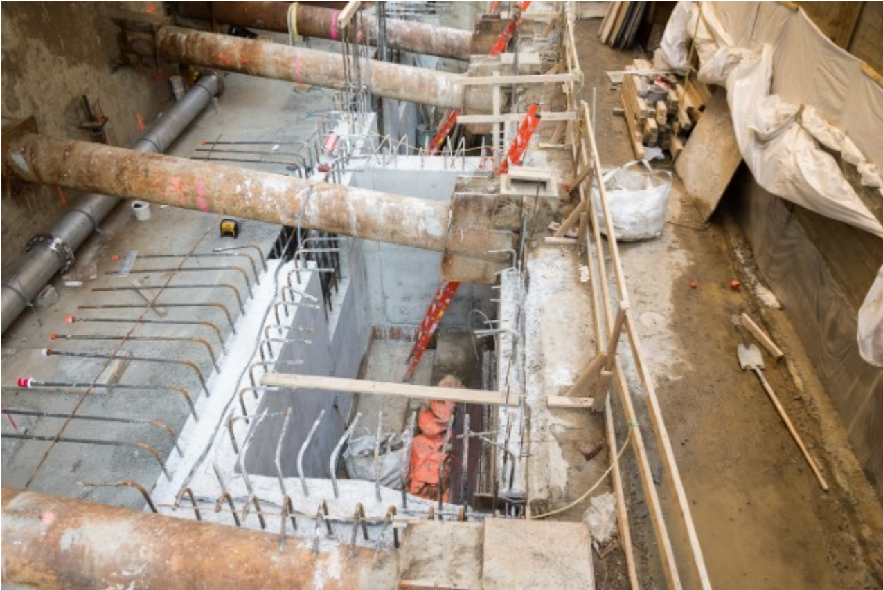
Photo of: North side/end elevator pit wall for slab to be poured on top of with concrete.
