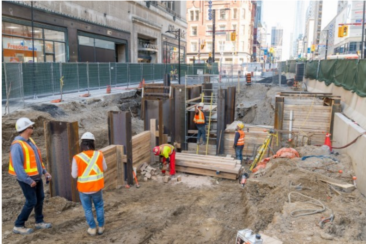
Photo of: Finger piles being placed on the north end of the site, to perform shoring support via timber piles.
