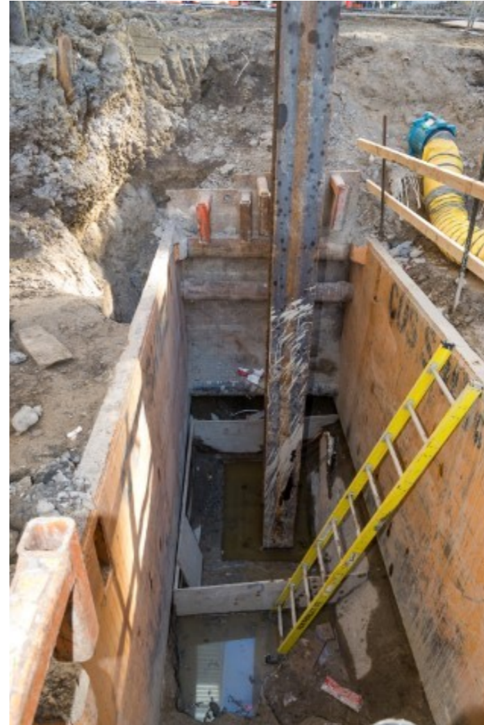
Photo of: Piles being placed in order to support foundation for newly implemented elevators in the elevator pits (2 elevators in total).
