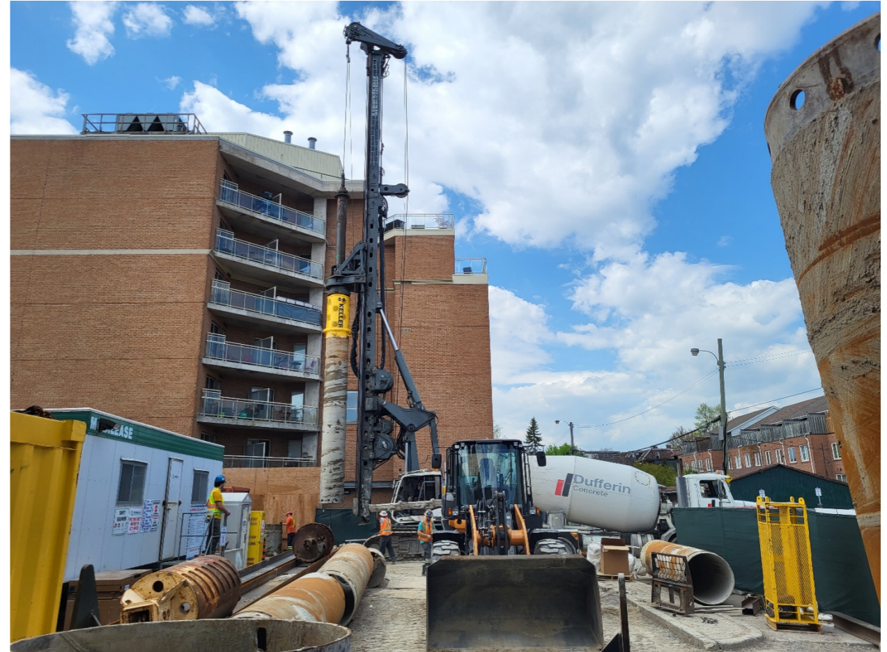
Drill rig and cement truck on the north side of Christie Station, looking north from Erlichman Ln.
