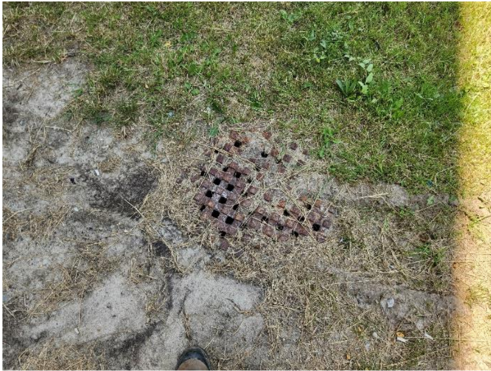
Image 25: Manhole in grassed area by Ellesmere Station, facing east.
