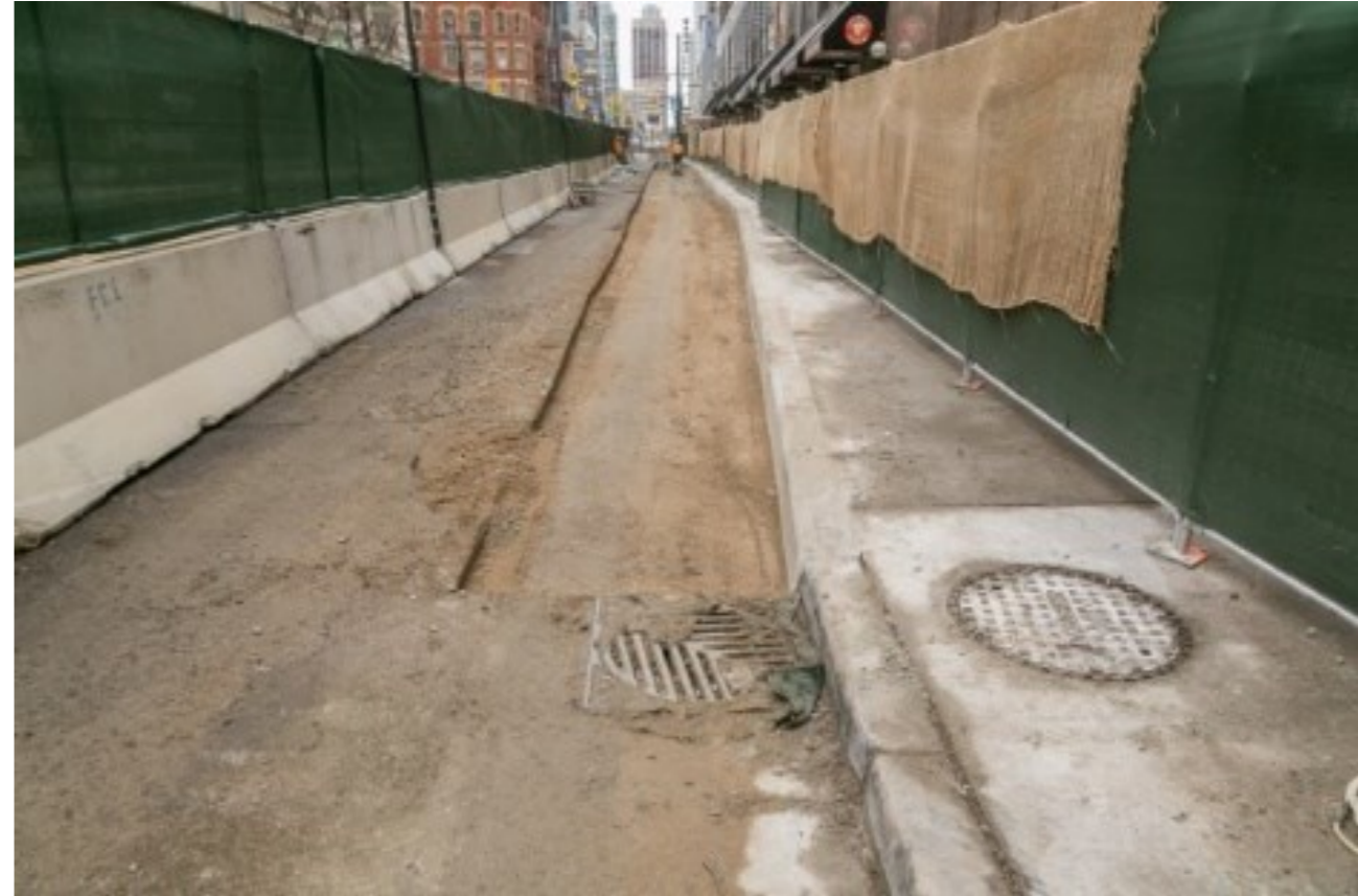
Stage 1A enclosure where Yonge St. is portioned in half while the other is being ready to be ripped up for start of construction.
