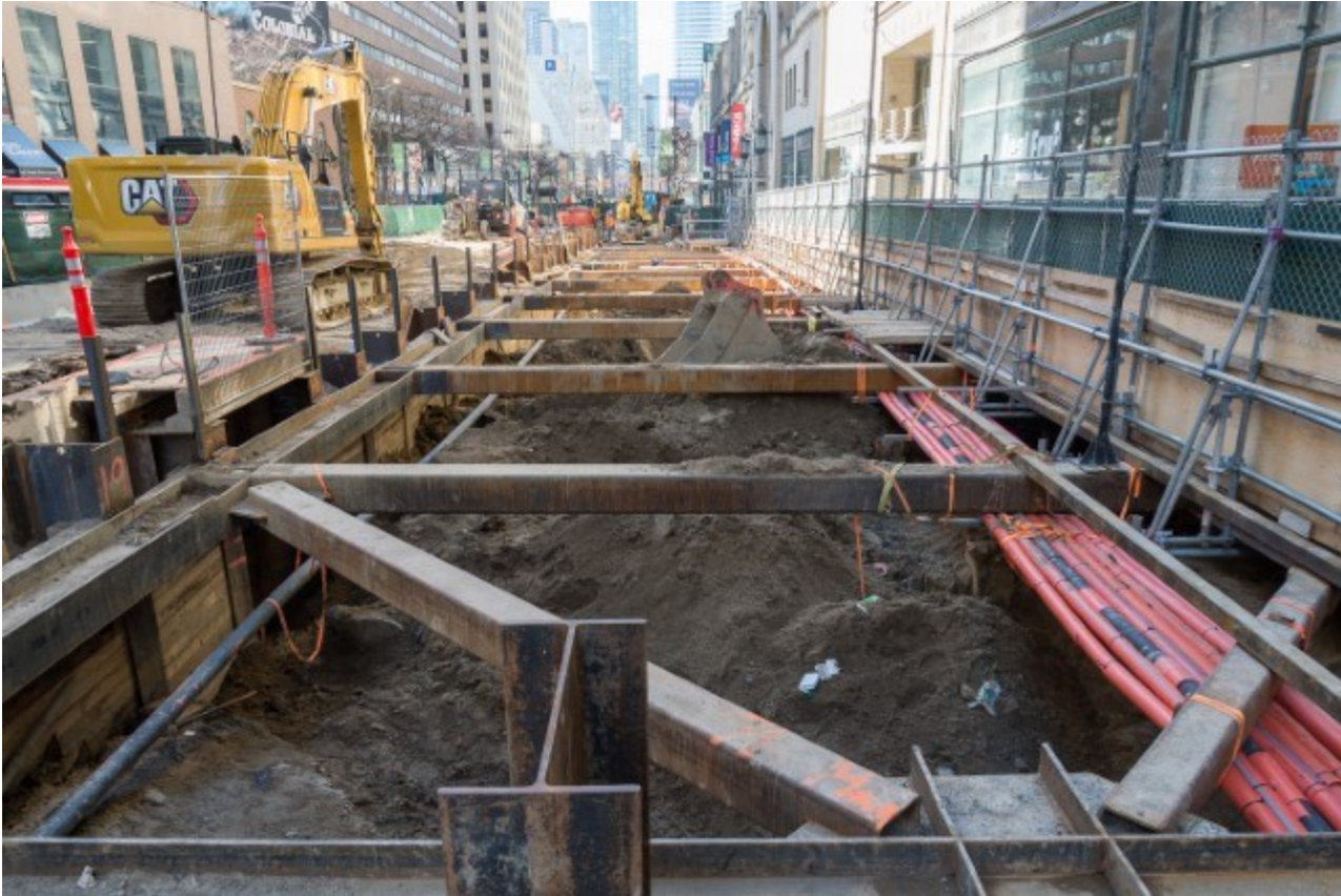
Walers, struts and horizontal hollow steel section beams in order to support shoring for further excavation.
