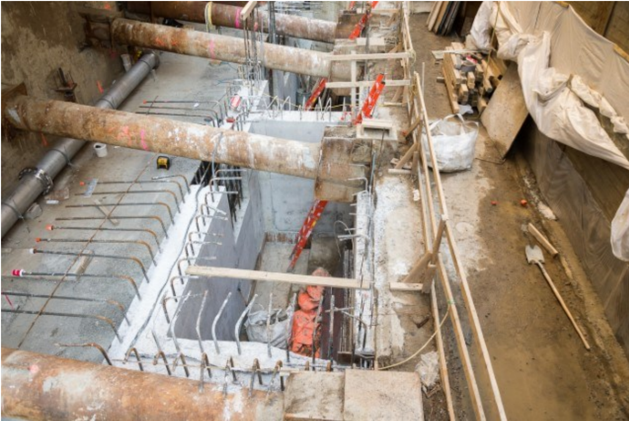
North side/end elevator pit wall for slab to be poured on top of with concrete.
