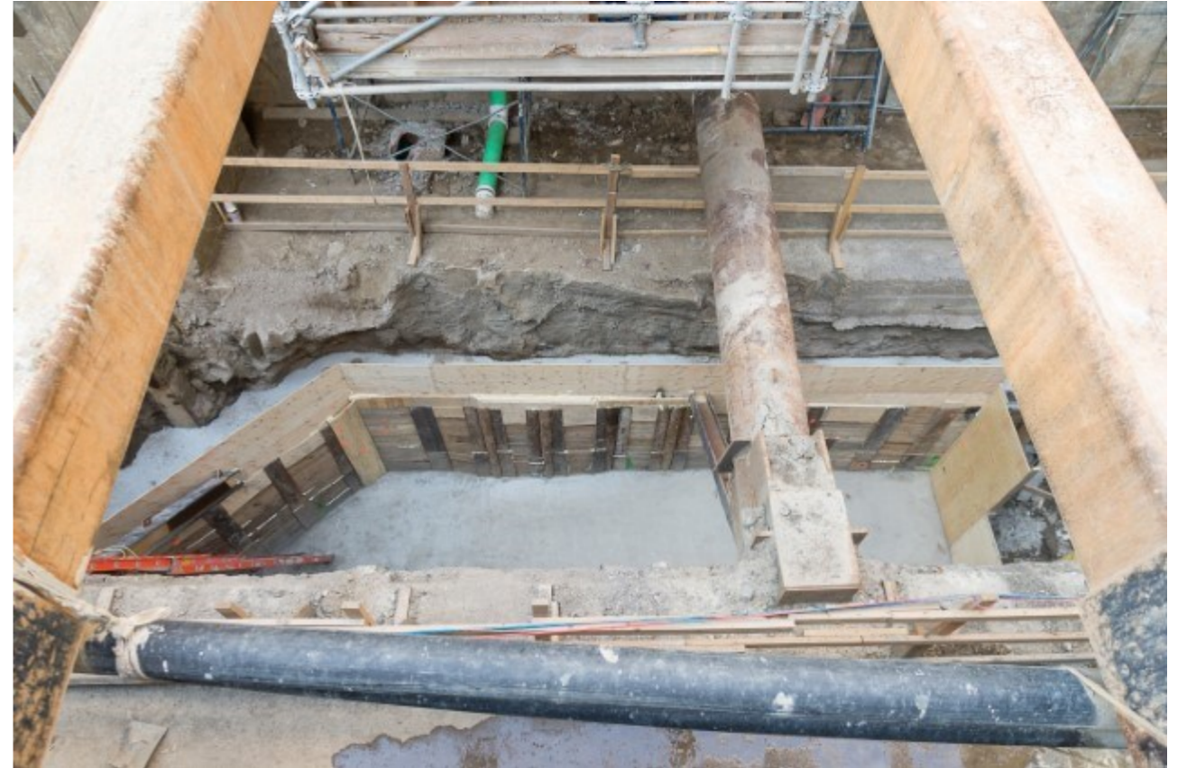
Mud slab at the south end excavation to aid in the development of new concourse and stairs from platform level.
