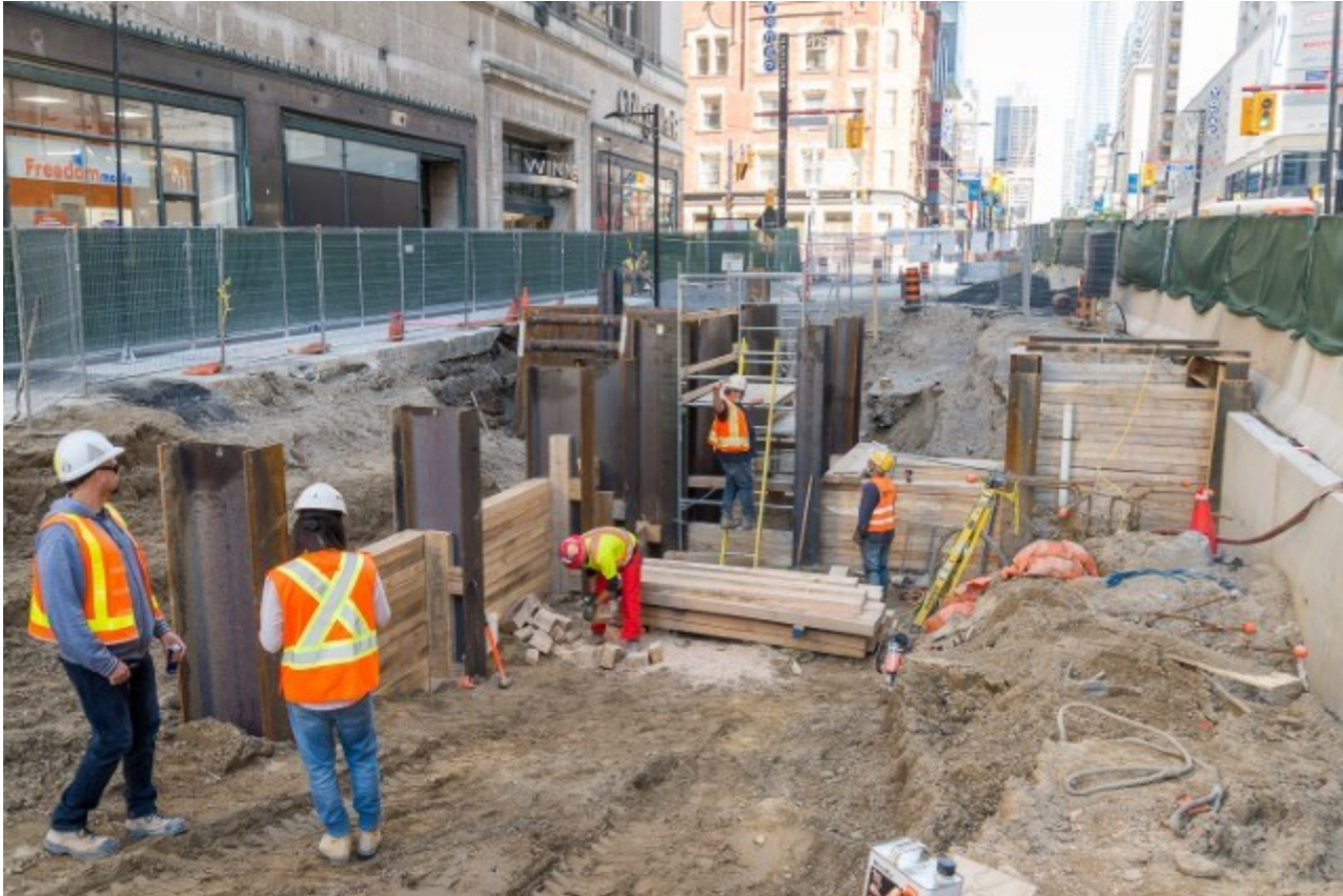
Finger piles being placed on the north end of the site, to perform shoring support via timber piles.
