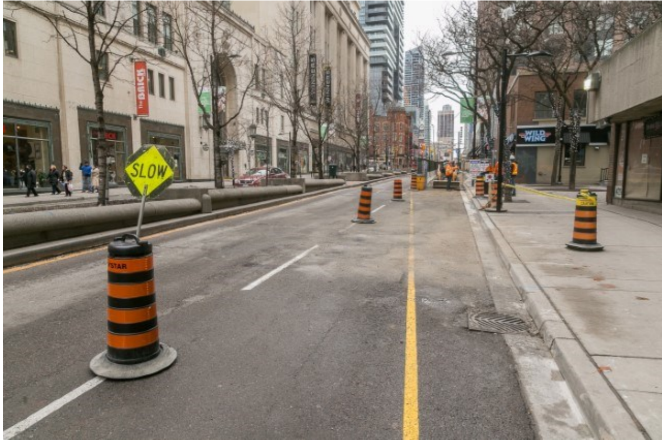
Staging traffic for safe access for workers to access initial work being done on curb.
