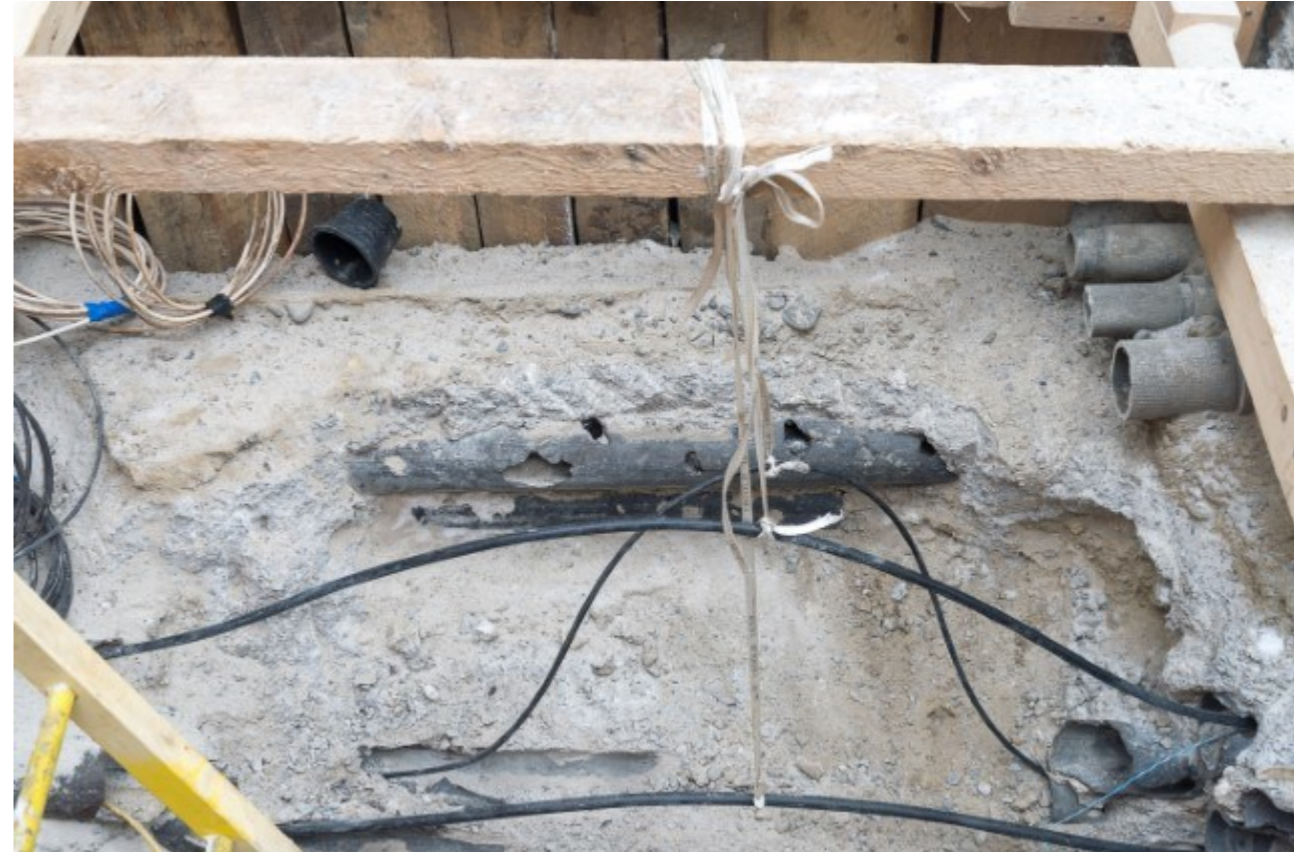
Exposed duct banks to be rerouted below ground – exposed conduits to be reattached and fitted with utilities such as telecommunications, internet, electrical etc.
