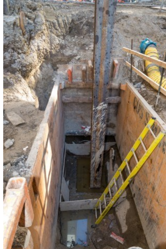
Piles being placed in order to support foundation for newly implemented elevators in the elevator pits (2 elevators in total).
