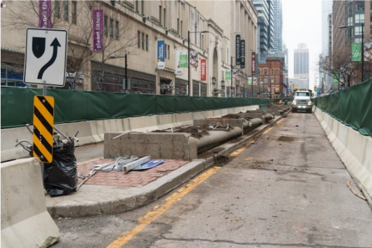
Median Demolition – median to be removed down Yonge St. in order to start Stage 2 demolition and excavation.
